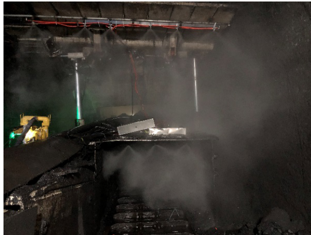
Figure 5. Spray effect of the return air lane.
